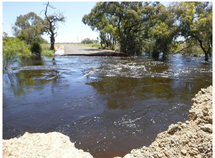
Wentworth Shire Council cut through Old Wentworth Road to alleviate the build-up of pressure on the Curlwaa levee from Tuckers Creek. Water was then directed naturally to Fletchers Lake.
