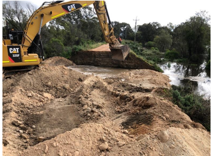
Section of levee breached on 19 November 2022 and was quickly repaired.
