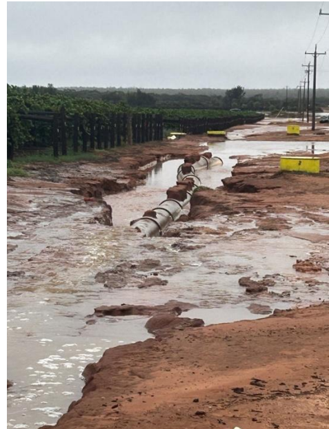
Coomealla Hollands Lake sub surface drain damaged by the record rainfall event 2 March 2026
